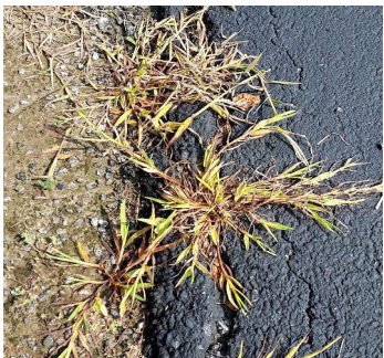
Wire grass breaking up the asphalt
